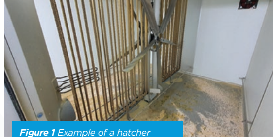
Figure 1 Example of a hatcher cooling coil covered with chick fluff.
