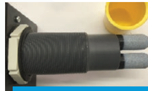
Figure 2 The photograph above shows typical CO 2 sensors in a setter, protected by sensor protection caps. If the caps become clogged with dust or condensation, the sensor will give an artificially high reading.
