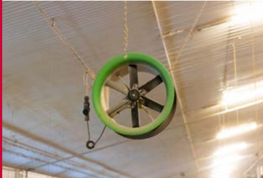
Figure 6.6 Circulation fans in an open-sided/naturally-ventilated house.
