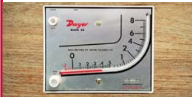
Figure 6.9 A manometer used to monitor air pressure within the house (the reading given is equivalent to 3.8 mm [0.15 in] of water column [37.5 Pa]).
