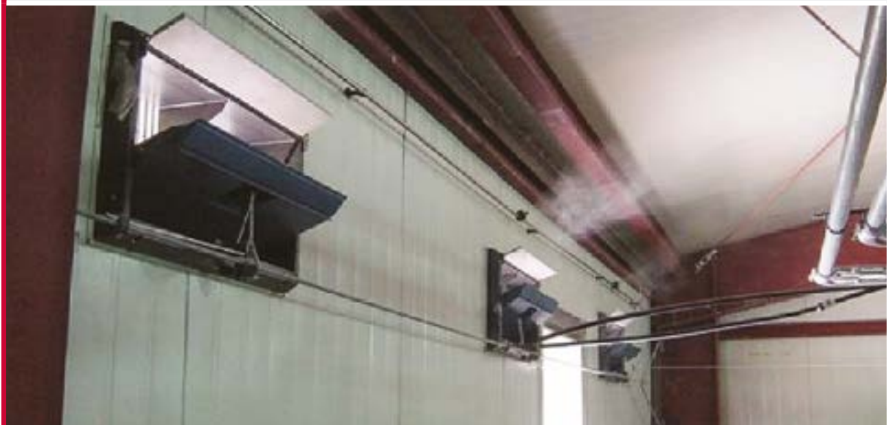
Figure 6.25 Example fogging system for a cross-ventilated house.
