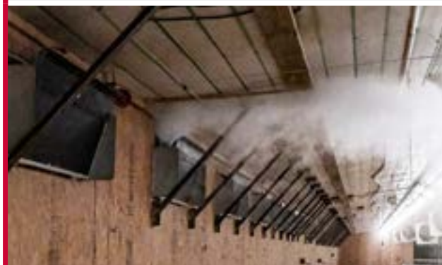
Figure 6.15 Using a smoke test to determine if air flow and operating pressure are correct.
